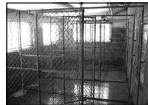
Mold growing where old roof meets newer roof.
